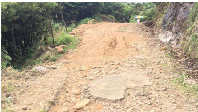
Poor condition of the access roads
